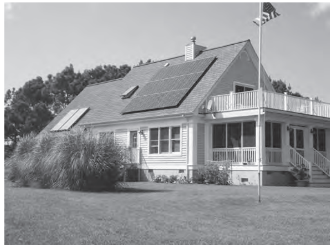
Our house with solar panels installed – two panels for solar hot water on the left, and 18 photovoltaic panels on the right. For scale, the house is 52 feet long (20 feet for the garage, 32 feet for the house).
